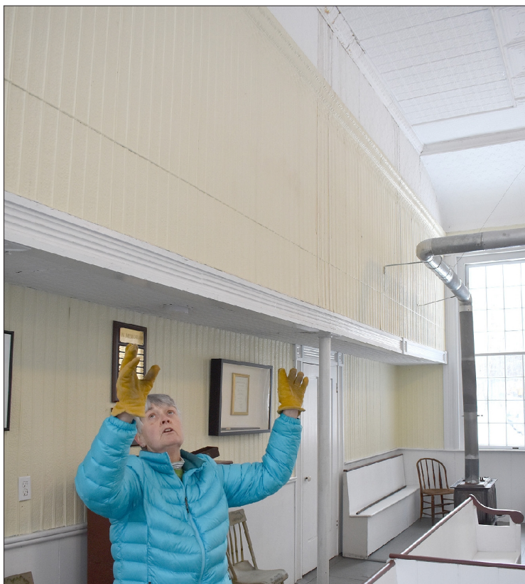
Susan Kelley LeClerc shows the part of the First Baptist Church of Lower Gilman where water would fall through the ceiling, leaving puddles on the pews and on the floors, before temporary repairs were made in 2018. More permanent repairs are needed, and there is structural repair also necessary. (Adam Drapcho/The Laconia Daily Sun photo)
