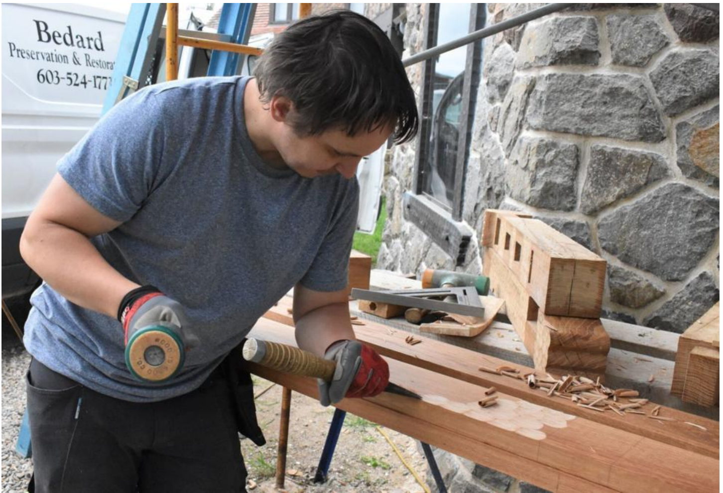
Thomas Juricka uses a mallet and chisel to chip carve white oak planks for the flooring of the balcony being replaced on the north tower. The balcony on the south tower was destroyed by a tree felled in the 1938 Hurricane, but has since been replaced with an exact copy.
